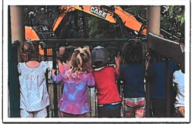
Children watch the geotechnical survey take place on the site of the future Early Learning Center in Bath
